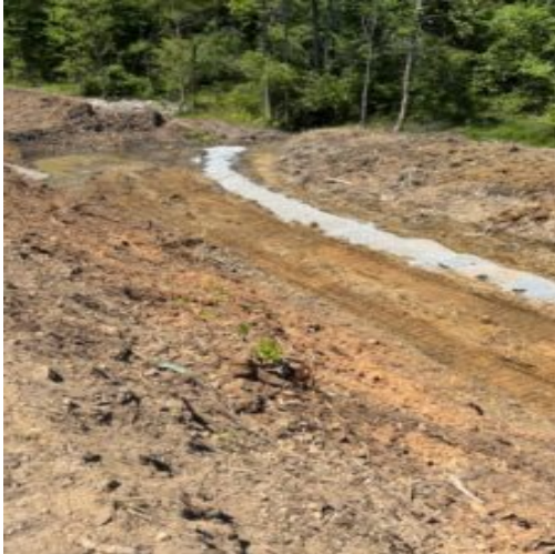
Installed drainage system approximately 105' long with #57 stone placed over top of wrapped filter fabric.
