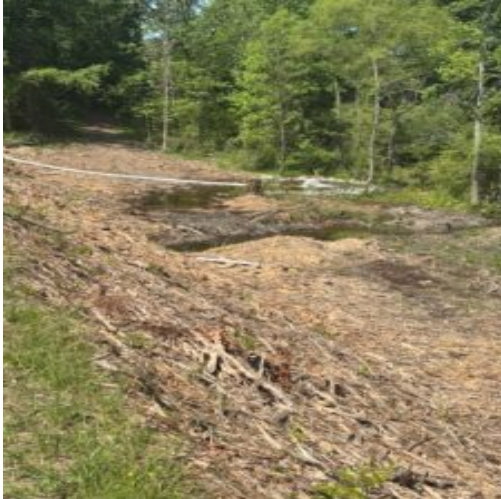
Wet area at toe of slope
