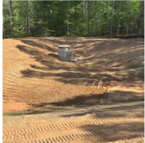
OCS at detention pond missing #34 stone at trash rack screen
