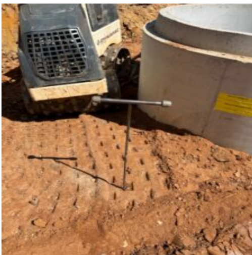
Backfilling, compacting and observation by probing using a rounded end steel rod
