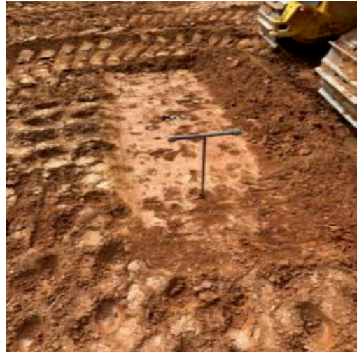
PM probing in place fill failed to meet required compaction
