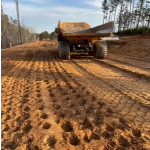
Proof roll indicating saturated soils in place with moderate movement
