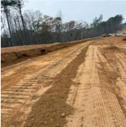
GAB placement area
