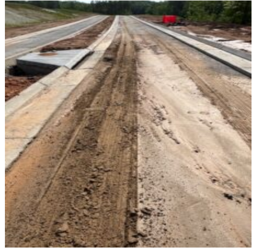
Washed silt over sub base stone
