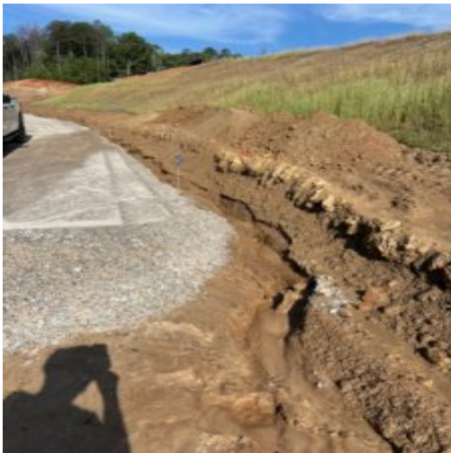
Gullies at curb line after rain event
