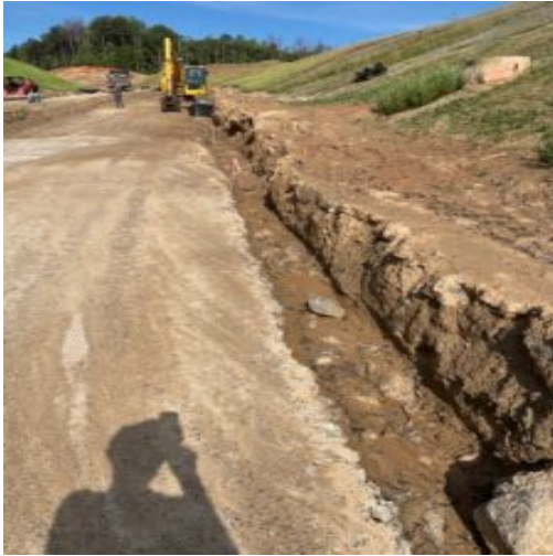
Washed gullies at curb line
