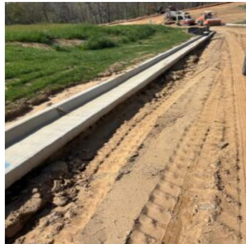
Washed eroded gullies at phase 1B
