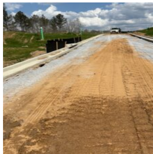
Base stone place at washed eroded gullies at curb lines unit 4 phase 1B
