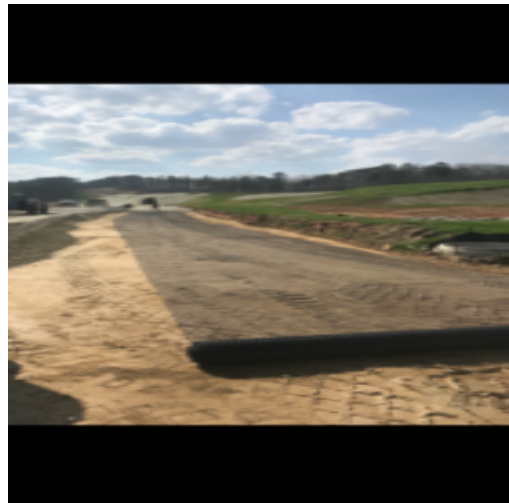
Tensor stabilization fabric (155'x13') place to stabilize subgrade between sanitary sewer manhole# 6 and 7 lower side
