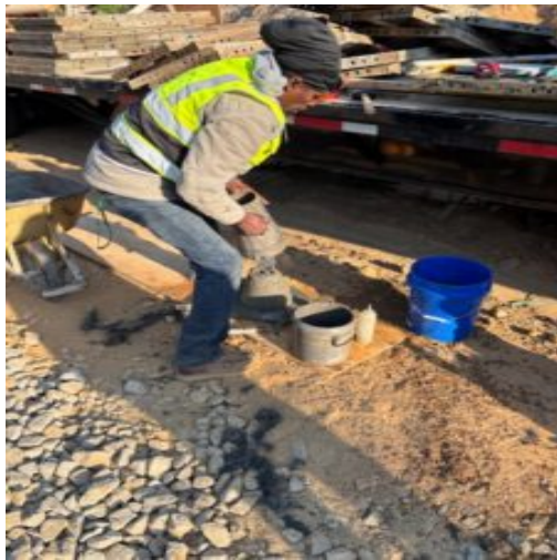
Performing slump test during concrete pour at north side bridge wall pour
