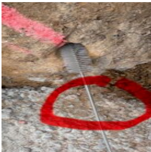
Fiber brush used to check cleanliness of drilled holes. Pulled out rock dust
