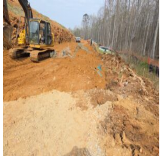
wall 1 contaminated area
