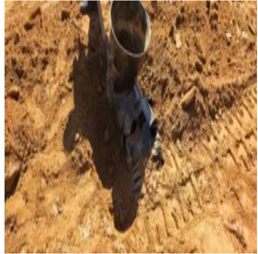
damaged drain wall 1
