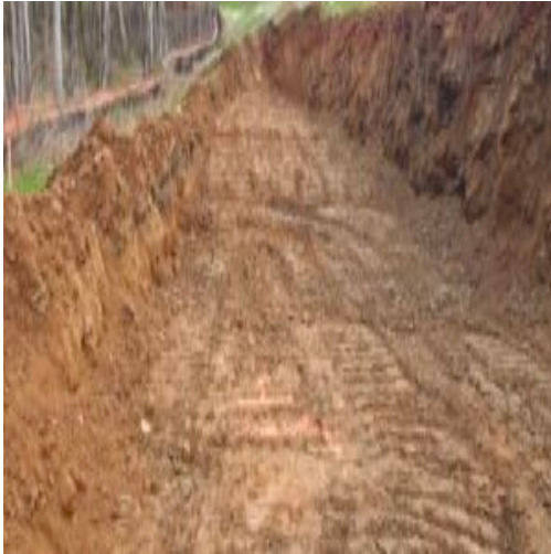
marked out soft spots on wall 1 footing
