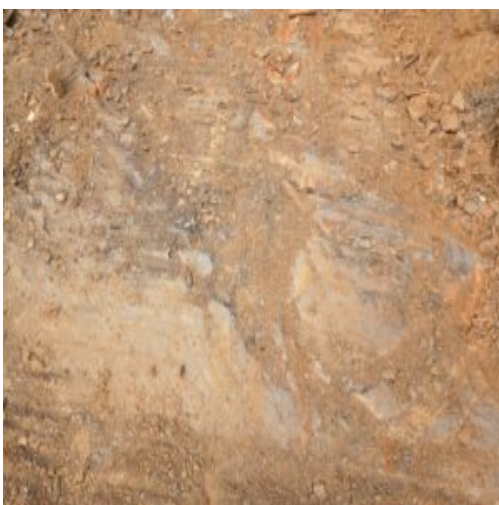
large slab of rock in footing of wall 1
