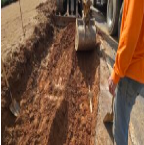
pipe found in lane extension
