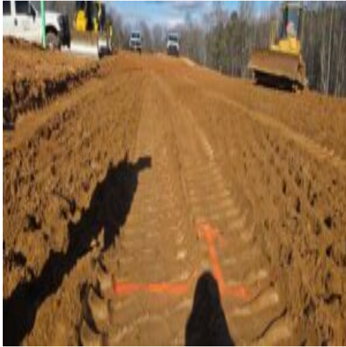
lots 30 - 32 pumping area
