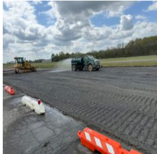
Increasing moisture on GAB
