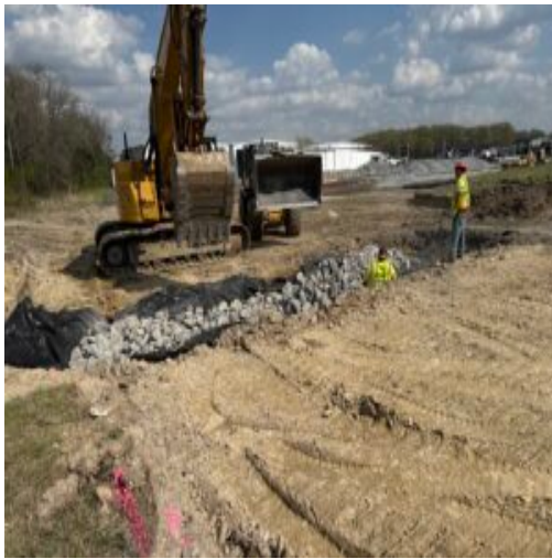
Large recycled rock placed into approximately 4 foot deep excavation on top of Geofabric. 40 x 15 feet
