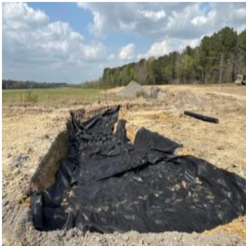
Geofabric placed inside approximate 4 foot hole due to large organics. 40 foot x 15 foot
