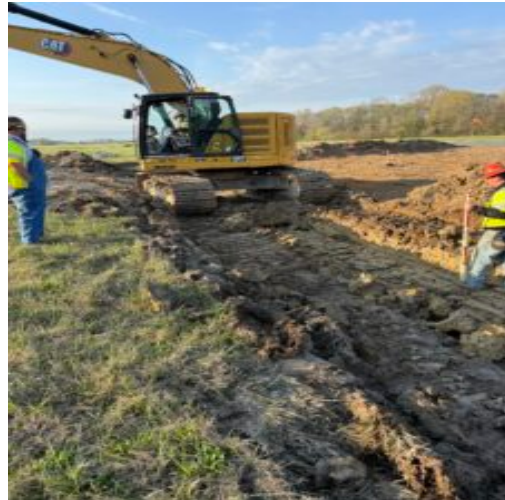
Storm drain undercutting
