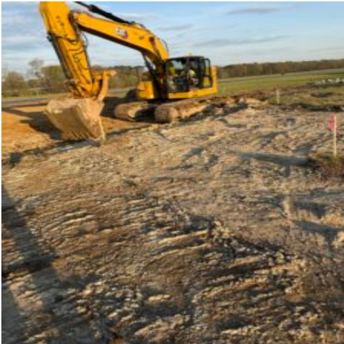
Storm drain undercutting
