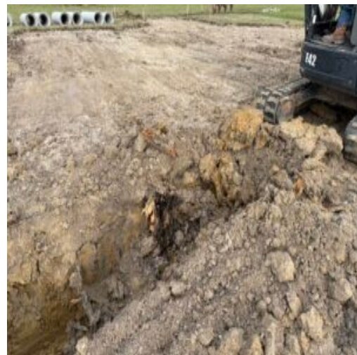
Duct bank trench with buried trees
