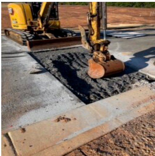
Undercutting in place base stone
