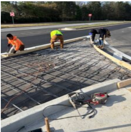
Observations being made of recommended repairs which were approved for concrete pour.
