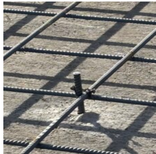
Drilled vertical dowels installed supporting the mat steel and prevent pour from shifting .
