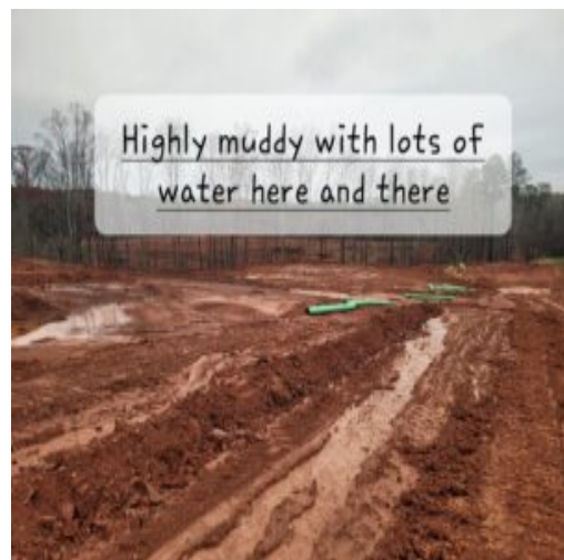
Photo depicting thick mud on both sides of the access road after the bulldozer move around
