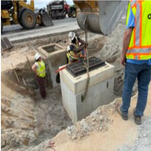
Area 1 box placement
